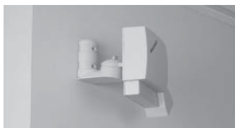
Small housing panel on MPAB11 wall mount
